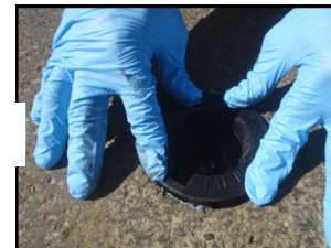
Place the SLT Base into the hole with arrows facing the direction of traffic (top surface is flush w/ ground).
