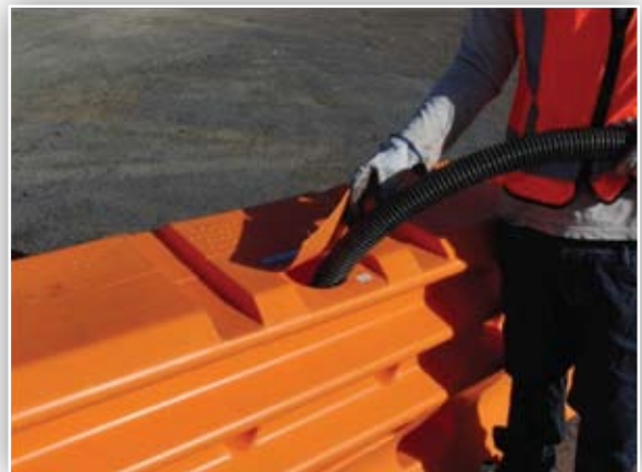
Figure 10: Using a truck mounted tanker fill each unit to the top with water.
