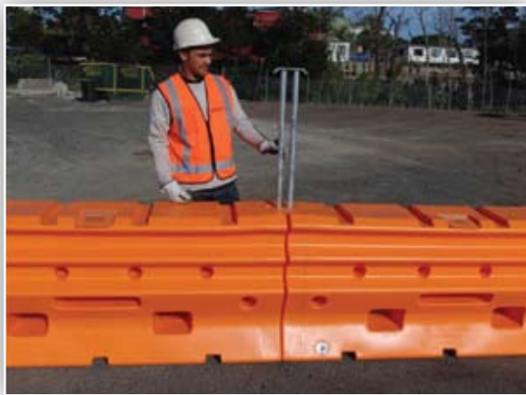
Figure 7: Once the units are aligned, the steel pin can be dropped into the alignment holes.
